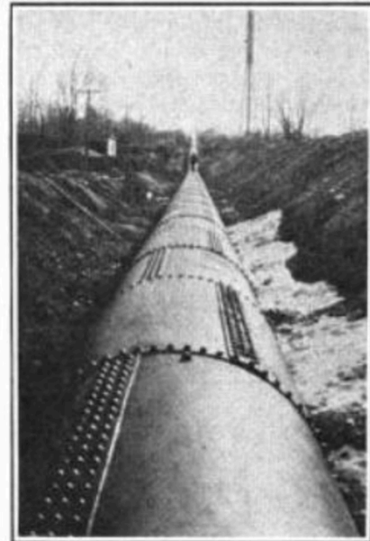
STEEL-PIPE LINE AND THE SURGE TANK, WHICH IS MOUNTED ON A TOWER
