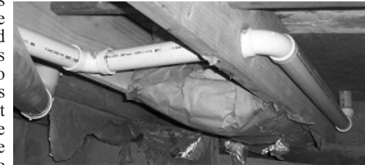
A small portion of the magnificent plumbing job. Get off my back about the insulation!
