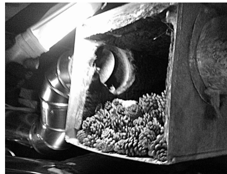
"The Nest" - New Duct Behind
